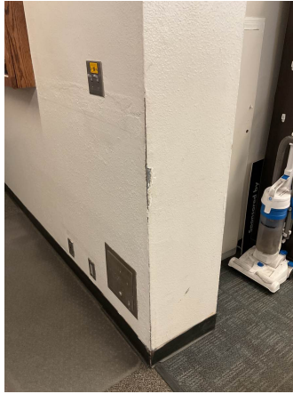
There is damage on wall corners.
