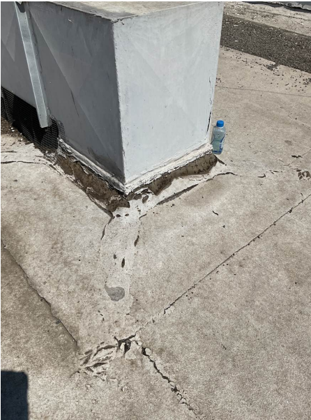
Several roof penetrations have sealant that are missing and should be replaced to avoid leaking.
