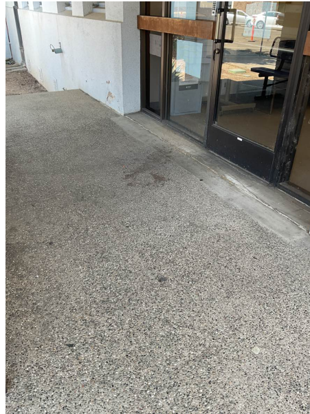
The front entrance has something spilled on it and needs to be pressure washed.
