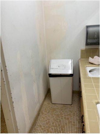
The men's locker room bathroom wall seems to have been repaired but not painted.
