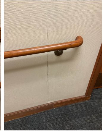
Sheetrock walls with wallpaper- several interior walls in the corridor have wallpaper peeling.
