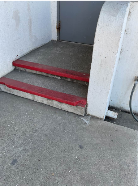
The steps on the west side of building have several areas that are chipped and damaged.
