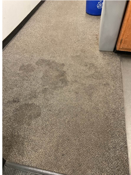
The common area carpet needs to be professionally cleaned or replaced.
