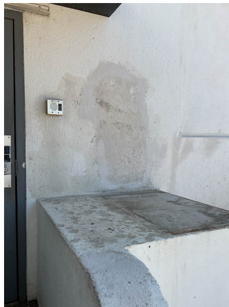
Stucco Walls- Several exterior walls are damaged, and the paint is peeling.
