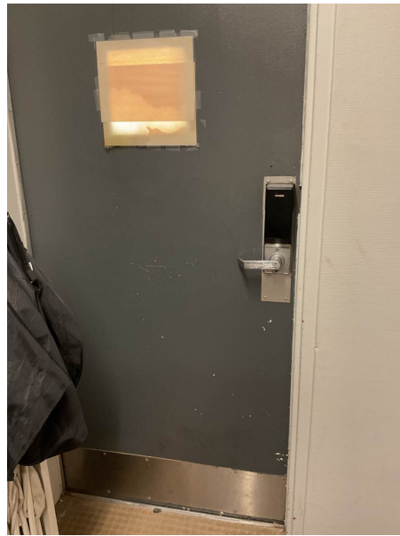
Glass/Metal Doors Several exterior metal doors are rusted and need paint and replacement.
