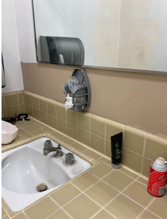
The men's locker room bathroom sinks are old and showing signs of wear. The soap dispenser is damaged and needs to be replaced
